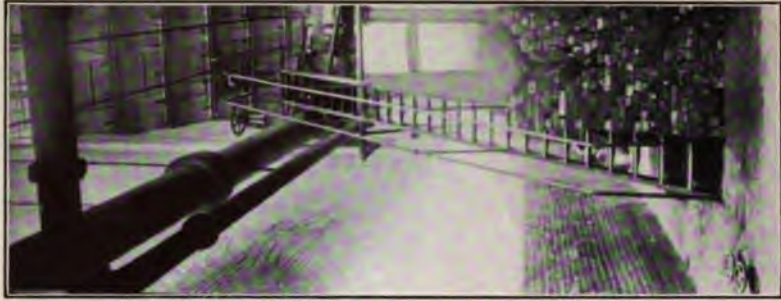
PLATE 2.—ANOTHER-VIEW This overhead cross walk of steel grating extends along the top of the boilers and gives access to each of the main valves.
